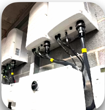
A new solar energy install in a south Manchester school
