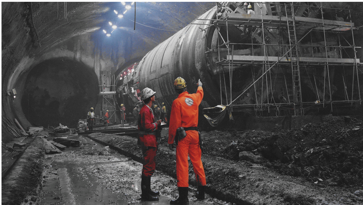
Figure 27 - Channel Tunnel UK undersea crossover cavern.
