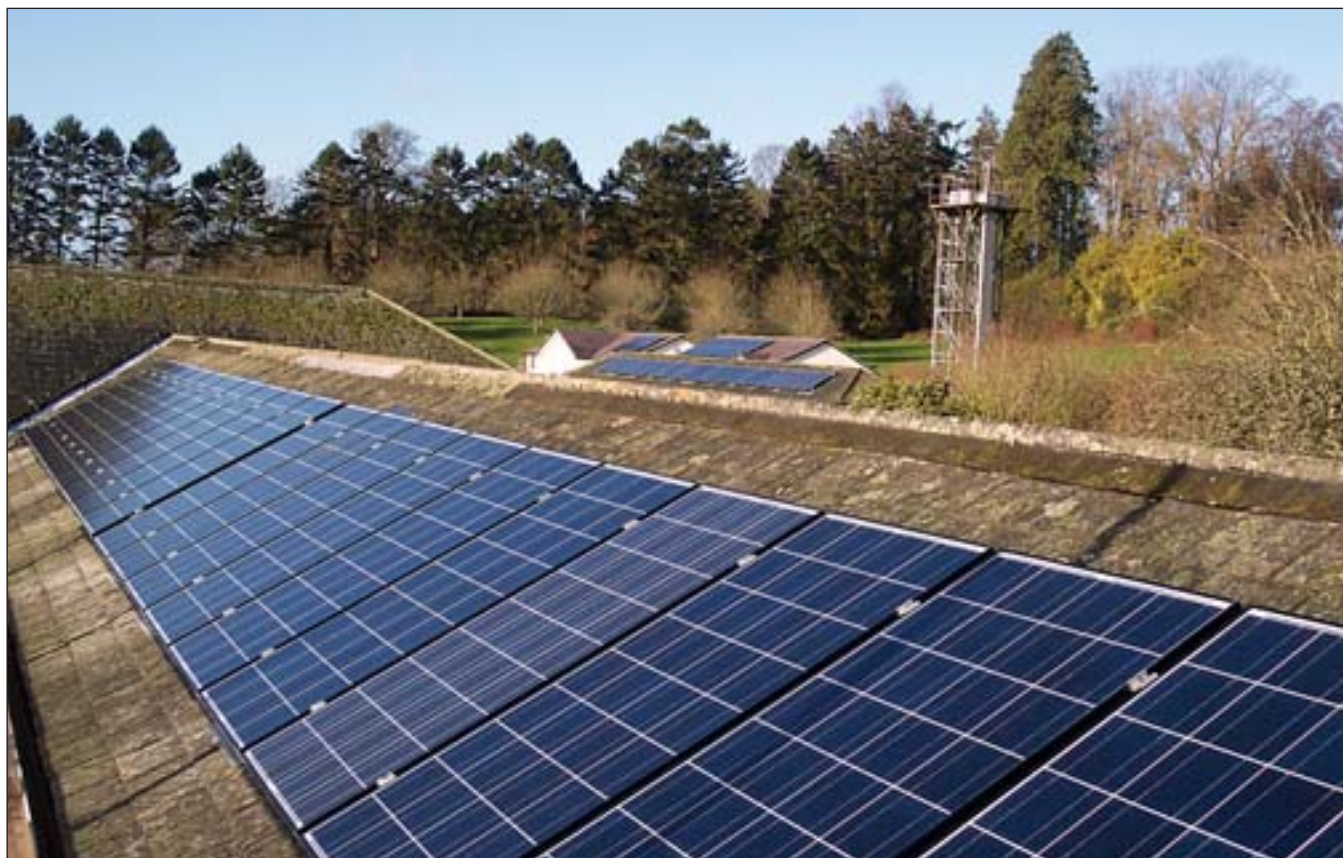
Photovoltaic installation at Bronllys Hospital, Powys. Courtesy of Powys Local Health Board and Welsh Health Estates
