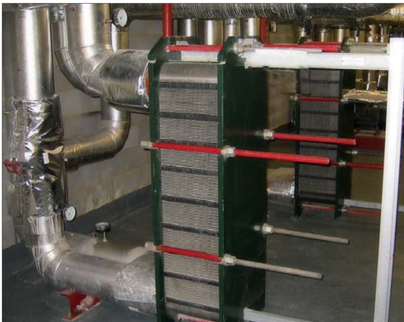
Princess Royal Hospital, Bromley. A view of plate heat exchangers in a plantroom at the Princess Royal Hospital
