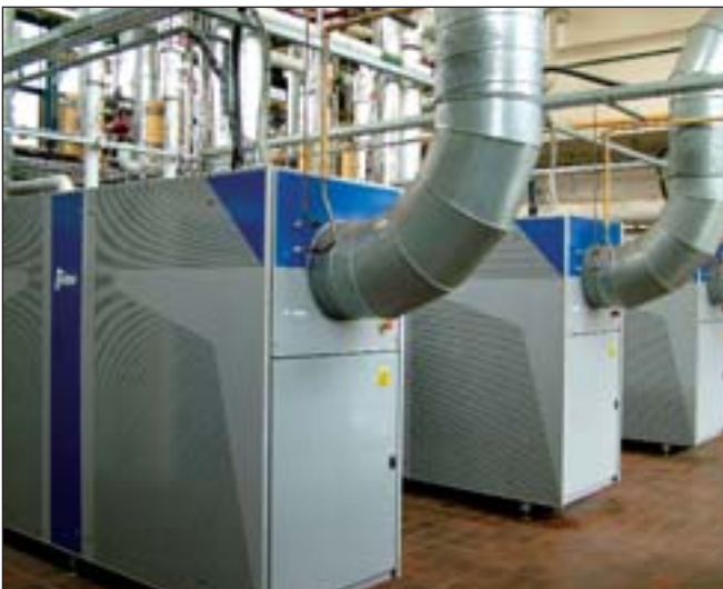
Nevill Hall Hospital, Gwent Healthcare Trust. Micro-turbine combined heat and power plant. Six micro-turbines – each rated at 100 kW electrical and 150 kW thermal output. The units can be sequenced much like a modular boiler installation. Electricity is used to offset import requirements and the heat output services heating and hot water demands in the winter and cooling in the summer
