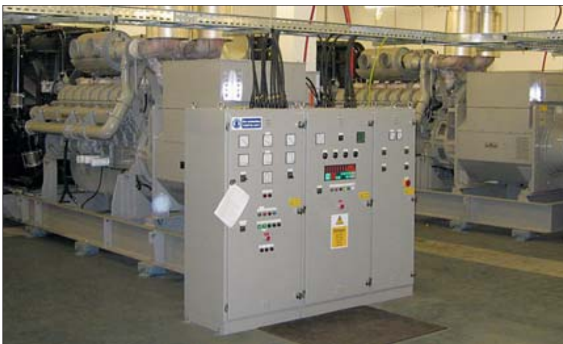
Princess Royal Hospital, Bromley. A view of the standby electricity generator plantroom showing good access space for maintenance etc
