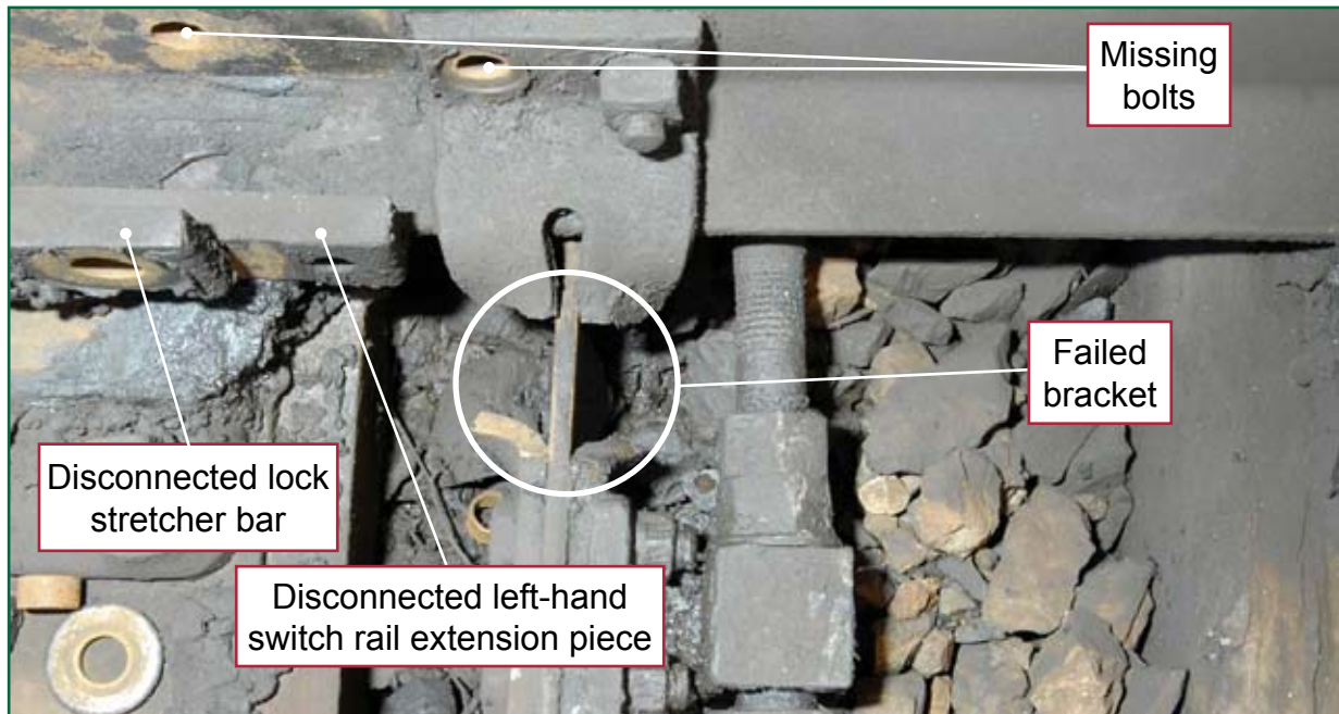
Figure 16: Failed bracket first permanent way stretcher bar
