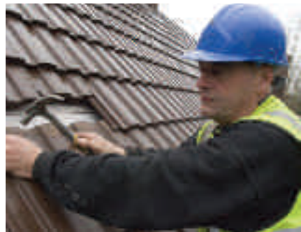
The 500 th new roof to be fitted under the 2007/08 SFA re-roofing programme
