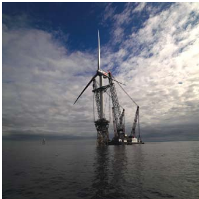
Installation of one of the two 5 MW turbines on the Caithness coast, Scotland.
