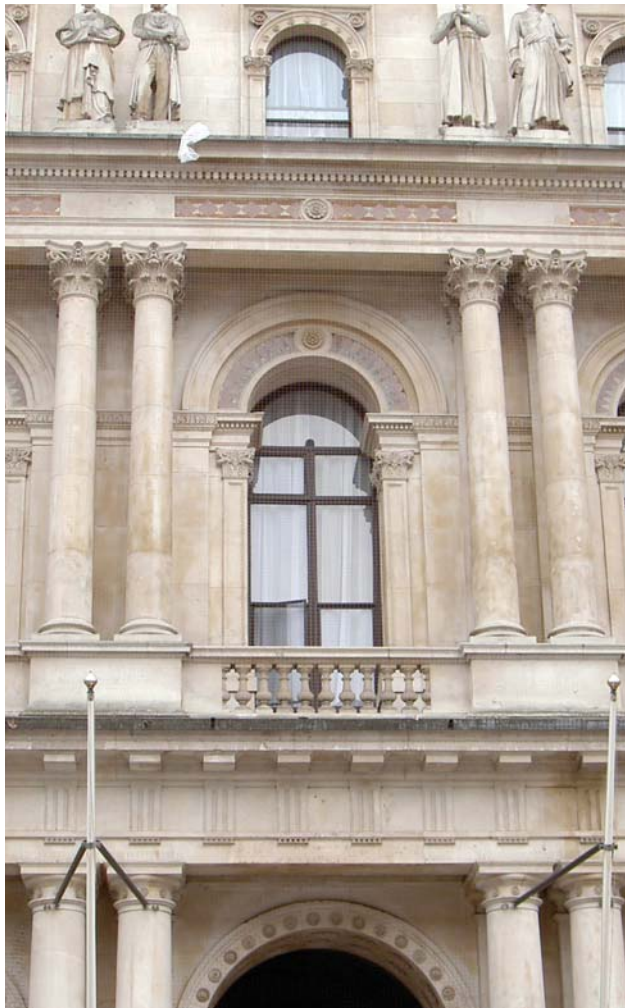
South elevation of quadrangle showing brown staining on columns
