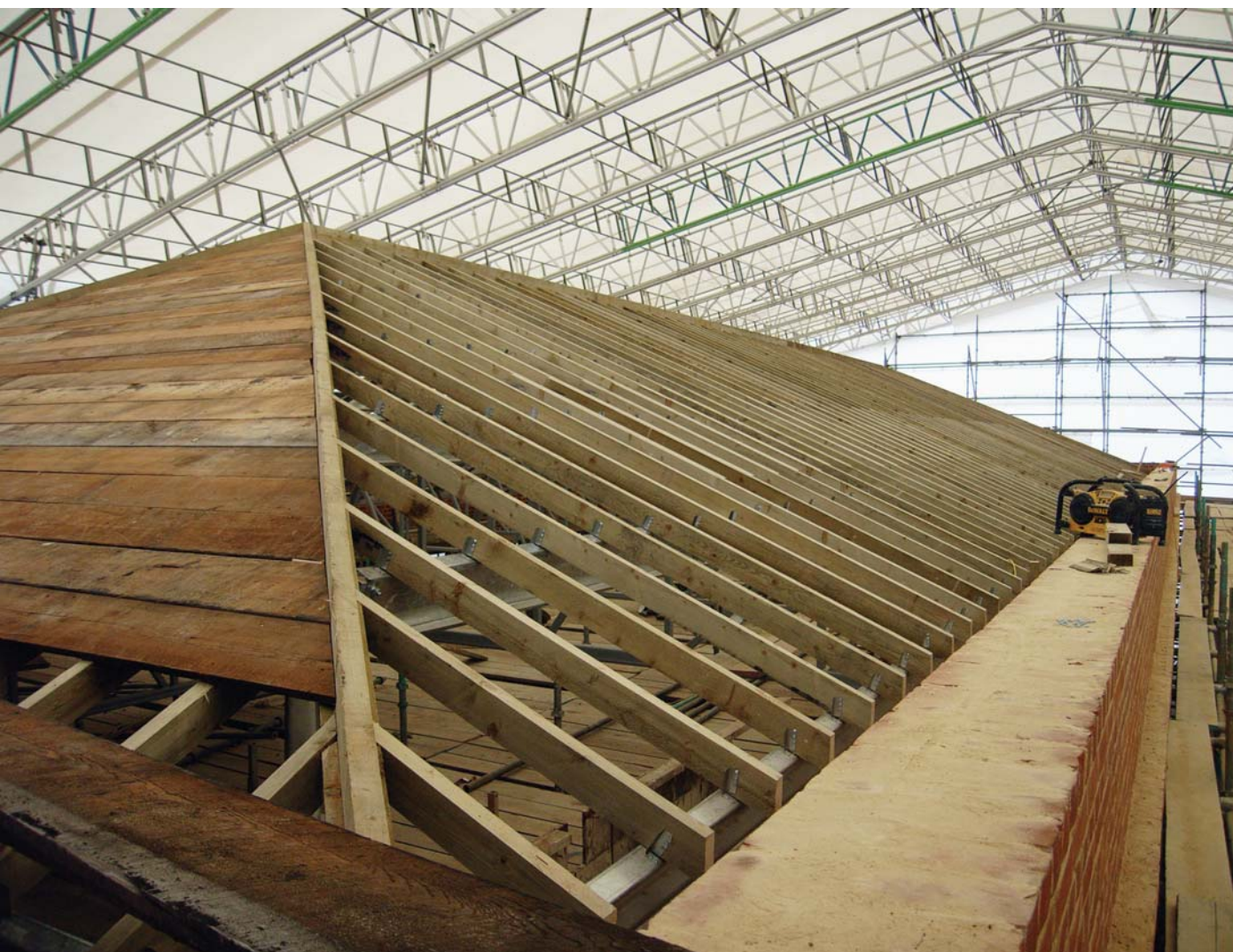
Work in progress on the new roof and brick parapets of the north wing of the Block Mills
