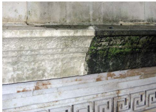
Results of DOFF cleaning on the south elevation of the quadrangle, before (right) and after (left)
