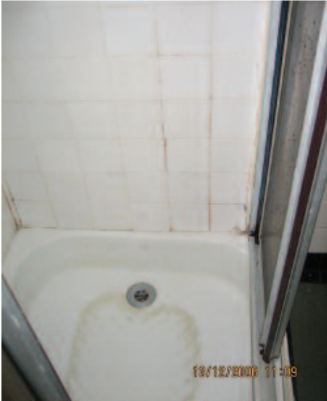
Photo 3: Dirty shower on ward 14a, Kent and Sussex Hospital (13 December 2006)
