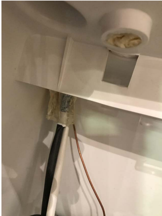
Photo 1 Foam fill point above Run capacitor
