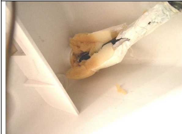
Photo 6 Untested foam around cable and capillary entry point
