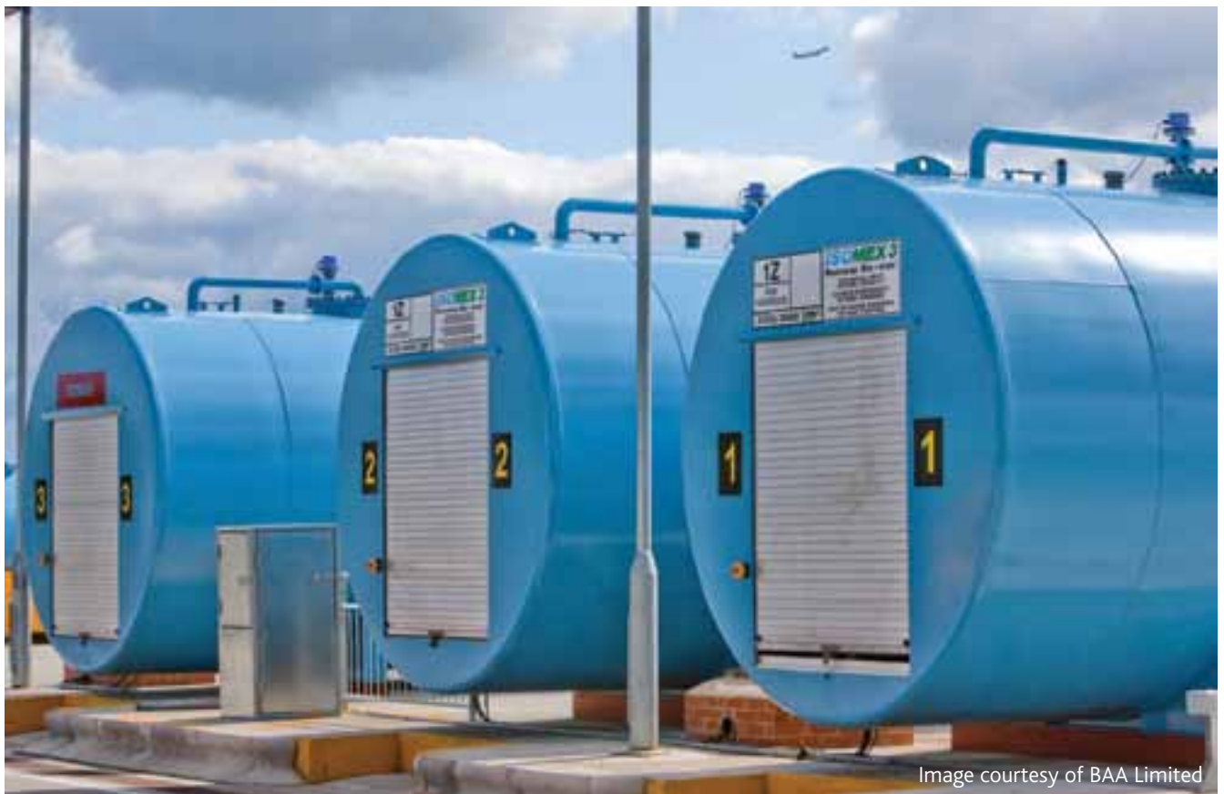
Figure 8.4 De-icing storage tanks
