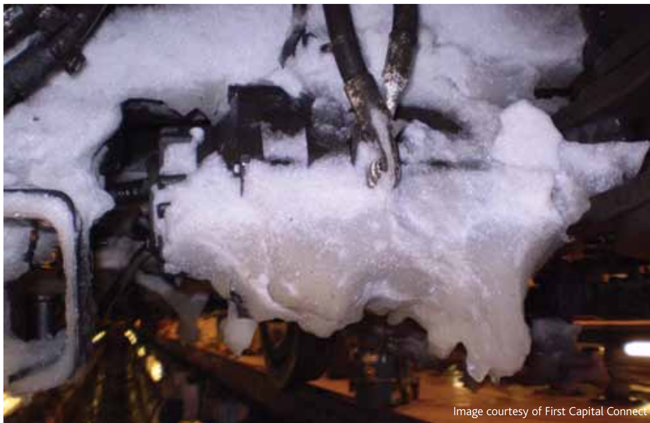
Figure 5.1 Damage to underfloor train equipment by snow and ice
