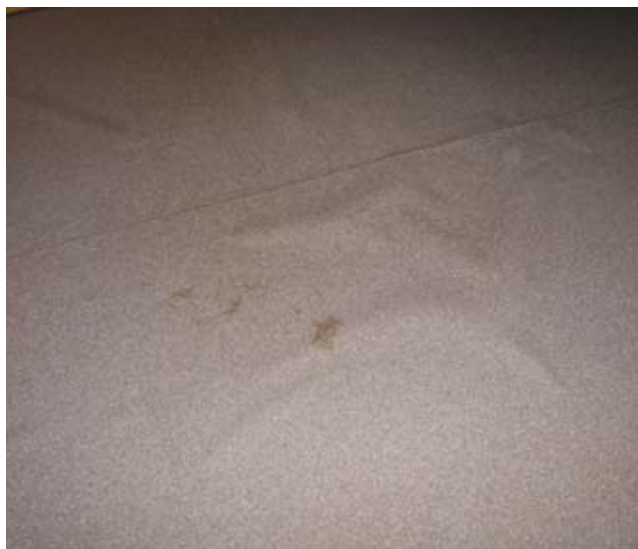
Good quality flooring material showing bubbles and wrinkles. Flooring problems are a common fault in new facilities
